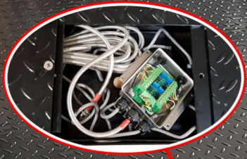
Top mounted Junction box
